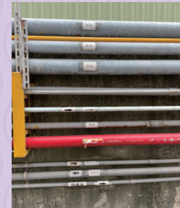
Pipeline tidying and labeling
