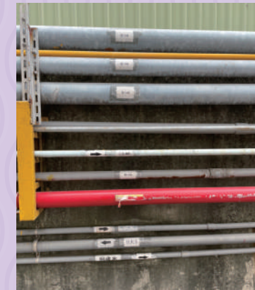
Pipeline tidying and labeling
